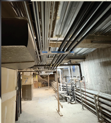
2" DoubleTrac® Dual Fuel Oil Supply (FOS) and Fuel Oil Return (FOR).
