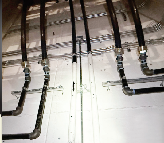
1-1/2" and 2" DoubleTrac® piping connected to steel pipe to the generators.
