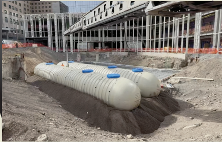
40,000-Gallon Underground Storage Tank.
