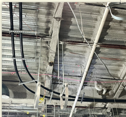
2" DoubleTrac® piping hanging on Unistrut Trapeze.
