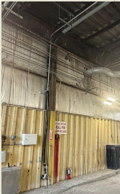
DEF-Trac® piping wall penetration and first sweeping turn at the roof.
