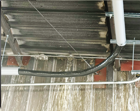
DEF-Trac ® piping second sweeping turn at the roof.
