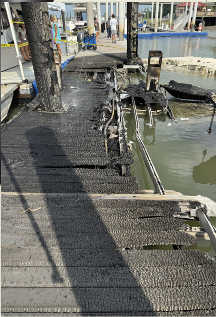
A major fire broke out at Palmetto Bay Marina on Hilton Head Island, South Carolina, resulting in extensive damage to multiple boats and surrounding marina infrastructure.
